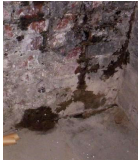
Cracks in basement concrete floor and brick walls
