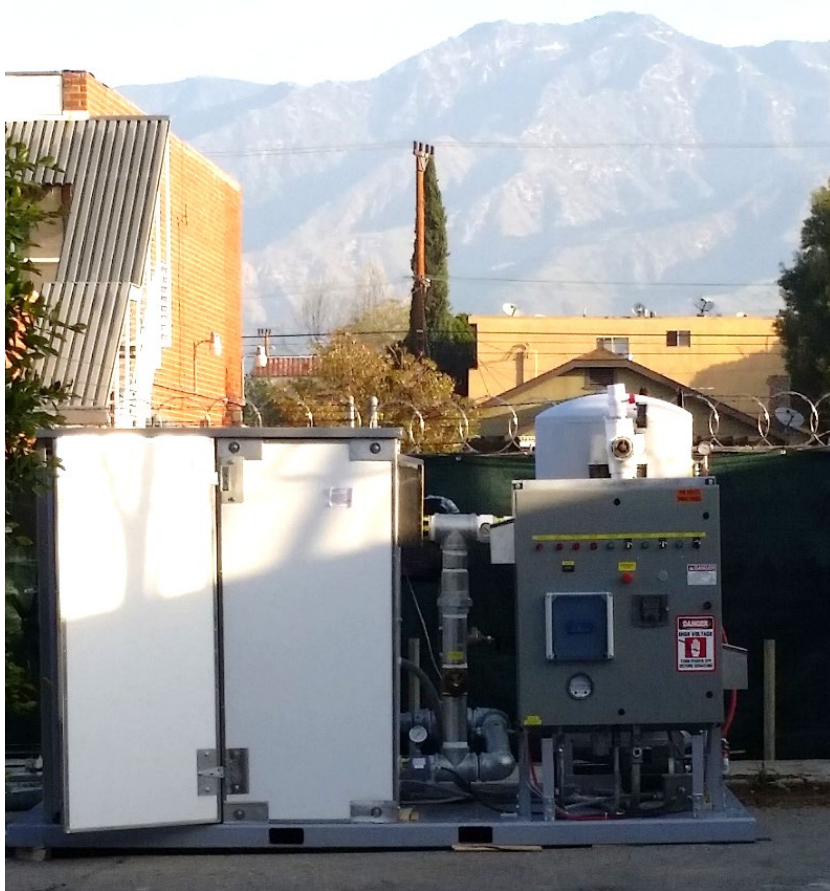
20-hp blower powered by a utility pole drop (up to 600 scfm)
